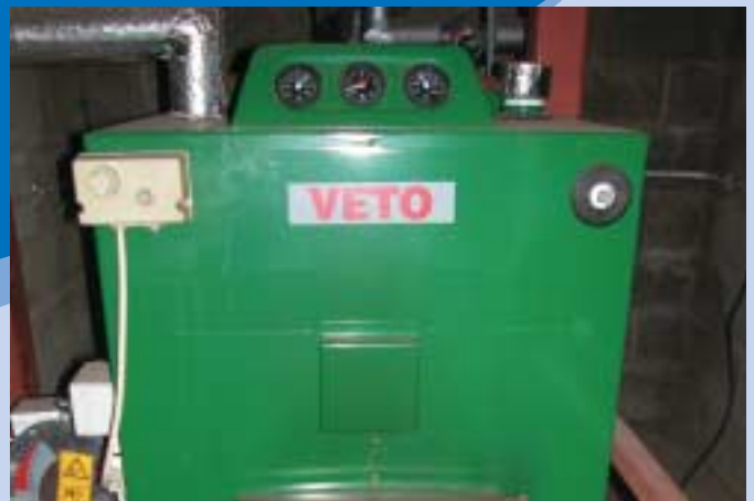
Hugh Buchanan's 60kW woodchip boiler
