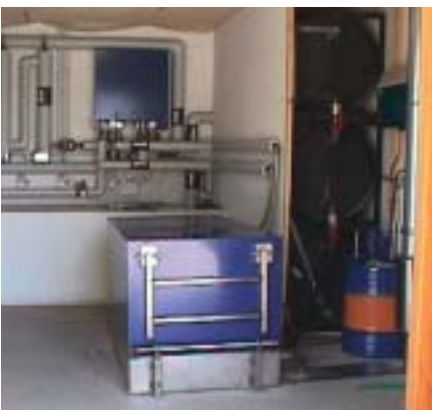
The plant room at Ramten, Denmark
