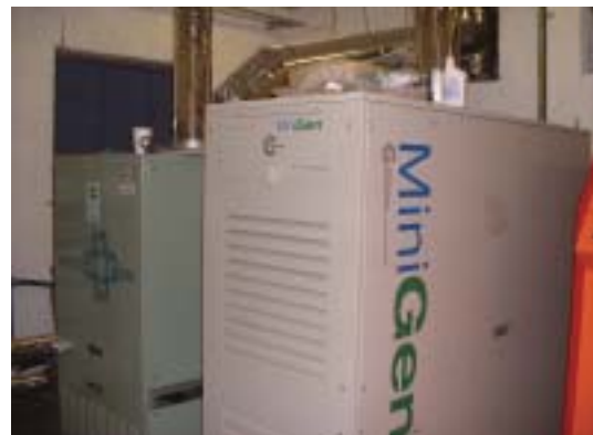
CHP unit at Weir Street, Cloch Housing Association.
